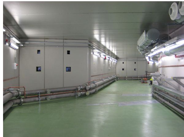
Fig.11: View of the tunnel which will host the Booster (right side) and the Storage Ring (left side).
