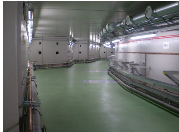
Fig.5: Inside the tunnel that will house the storage ring and the booster. The square holes visible on the concrete walls are for alignment (top) and for the exit of the synchrotron beam (bottom). The tubes at the left hand side are the cooling lines for the magnets of the storage ring. The first semicircle has already been cleaned and it is ready for mounting magnets and vacuum chambers. The large ducts on the upper right hand side belong to the climatization unit. The right angle brackets attached to the right wall are the supports for the bending magnets of the booster. Below them, the cable trays and water cooling lines are visible. Date: 2 Dec 08
