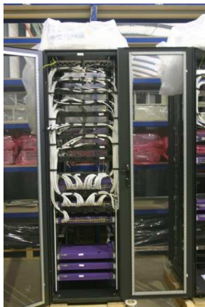
Fig.27: One pre-installed rack
