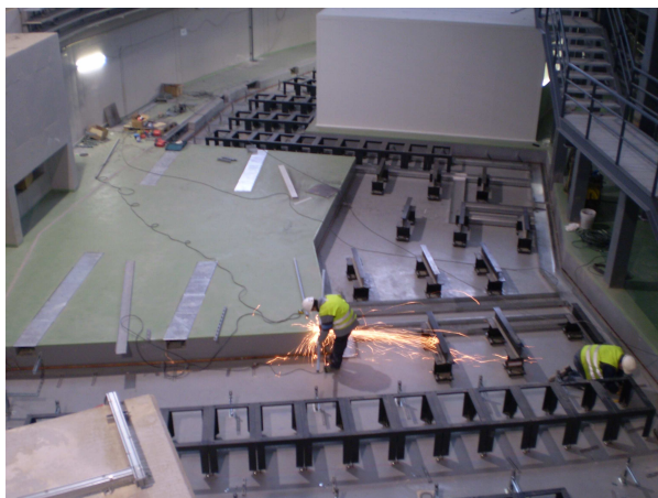
Fig.3: View of the service area at the inner part of the storage ring tunnel. The workers are installing supports for the cable trays that will be connected to the electronic racks mounted on a false floor on top of the metallic structures of the photograph. Date: 2 Dec 08
