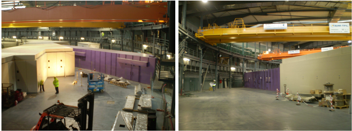
Fig.6 and 7: Views of the experimental hall during the preparation of the installation of the safety hutch of beamline 13. The photos also show the safety hutch of BL 11 (violet) already finished and the two orbital cranes .Date: 2 Dec 08
