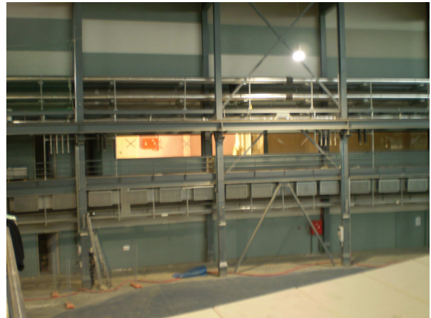
Fig.4: The Control Room, illuminated in the photograph, is located in the first floor above the Experimental Hall. The photo also shows the peripheral pipesthat will carry demineralized water to the beamlines r for cooling purposes. Date: 2 Dec 08
