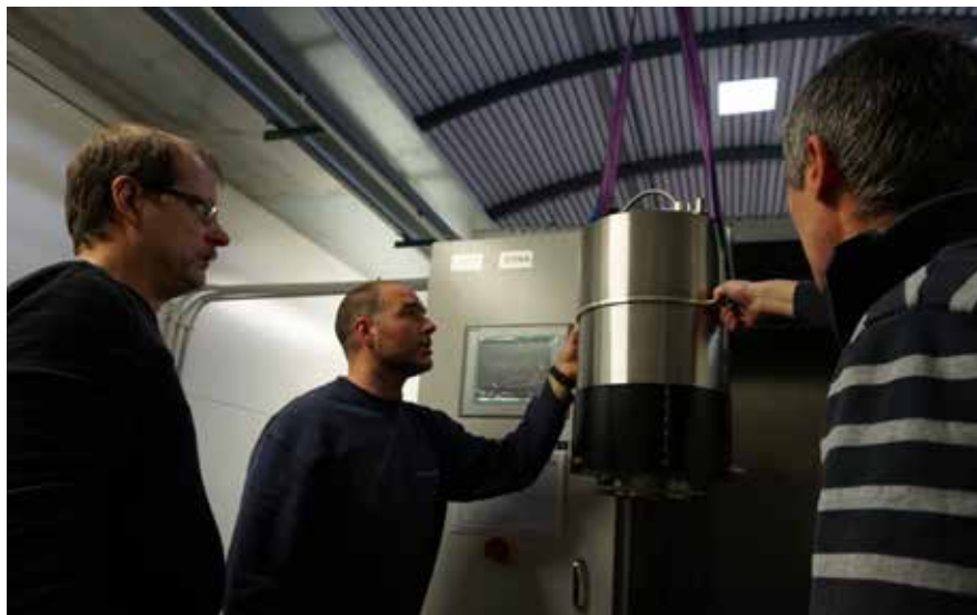
Installation at the RF lab of a new IOT, by ALBA personnel under the supervision of a company expert. © ALBA
