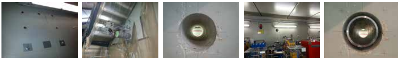
Figure 4: Sequence of images of the tunnel wall drilling done in December 2014. © ALBA Engineering division
