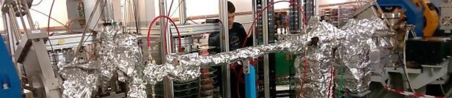
Inductive adders installed next to the stripline in the ALBA Storage Ring tunnel.
