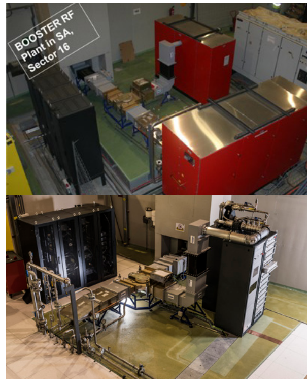
Old tube based Booster RF power system (top), and the new SSPA one (bottom).
