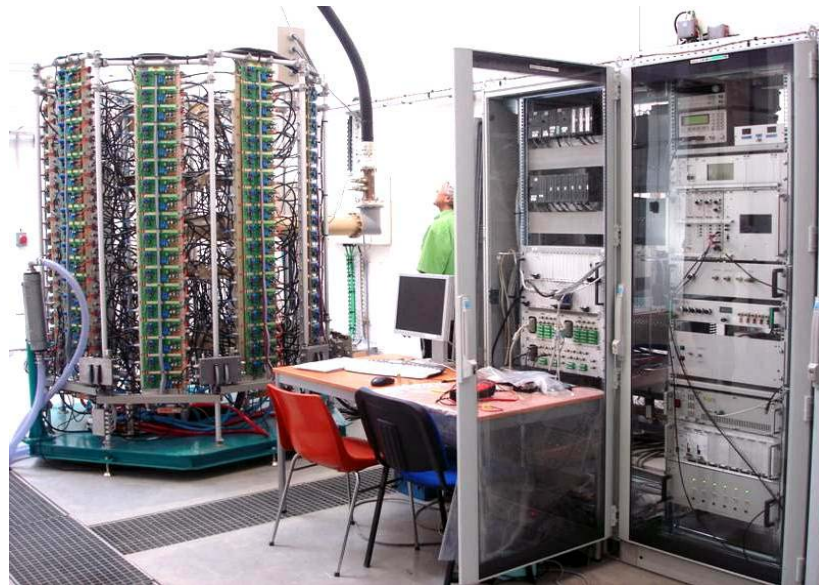
BO RF room (amplifier with LLRF & control)
