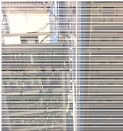
Power supply 50 kV, 200 mA
