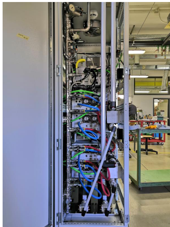
RF drivers connections ( cooling water- RF and PS) ready
