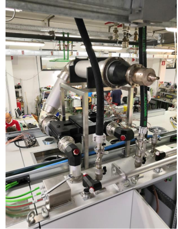
RF high power combiner ready on the RFPS roof
