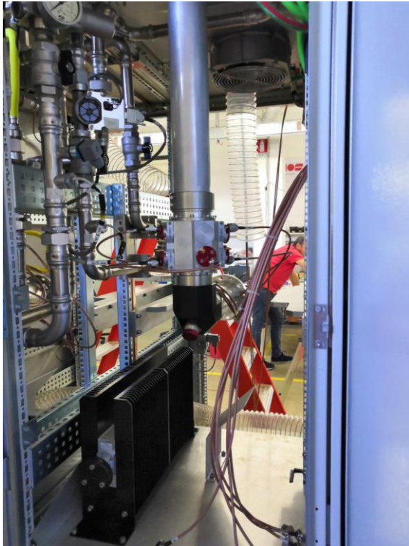
RF distribution for the tetrode ready
